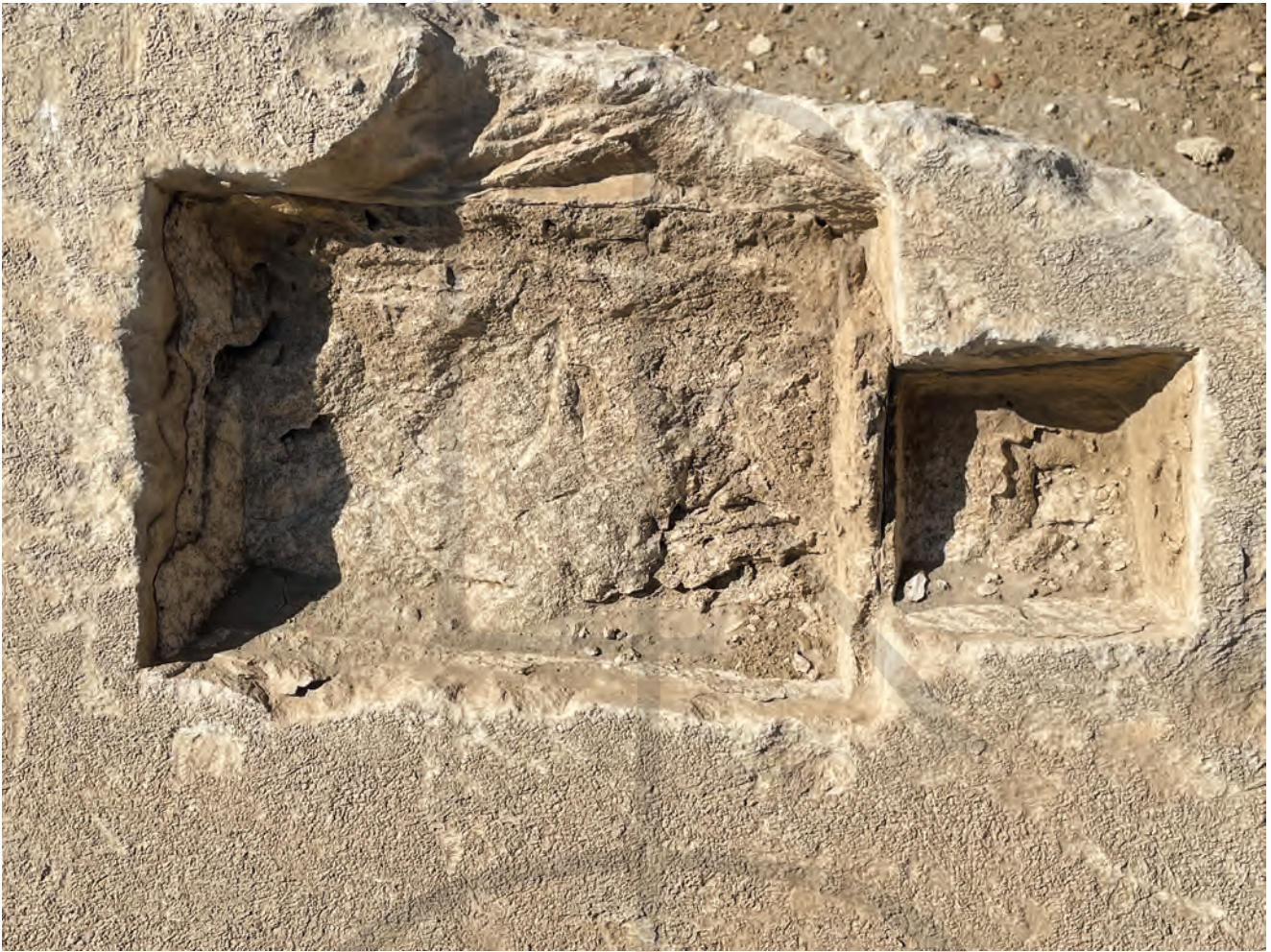
Fig. 2 Pyramid of Senwosret III. Sockets for multiple patch stones in the casing. (Photo D. ARNOLD)
