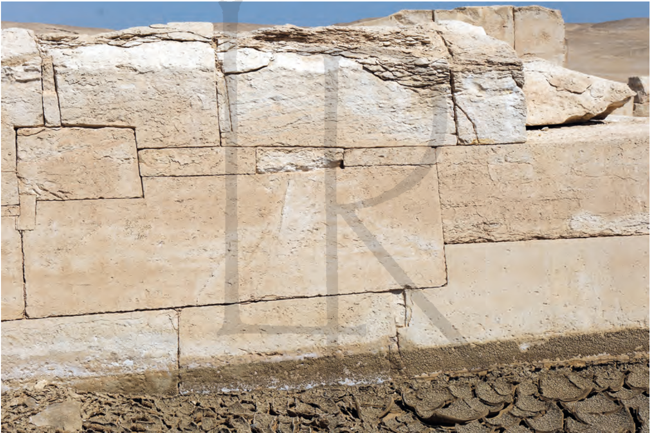
Fig. 10 Valley temple of Snofru. Damaged south wall with patch stones. (Photo D. ARNOLD)
