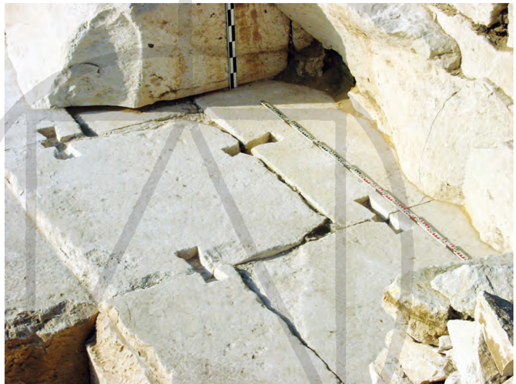
Fig. 8 Pyramid of Senwosret III. Casing blocks connected with multiple dove-tail cramps. (Photo D. ARNOLD)
